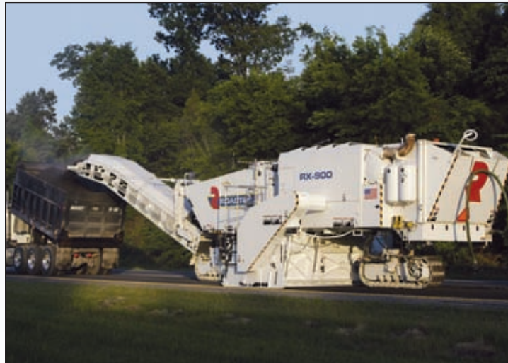
LoJac Enterprises, Inc. of Lebanon, Tennessee does a lot of paving work with hot-mix asphalt (HMA). LoJac has eight pavers, three milling machines, and three Shuttle Buggy material transfer vehicles (MTVs). The availability of replacement parts is obviously a key factor for this company.
