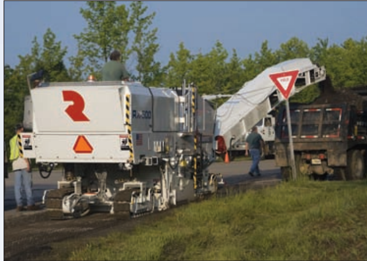
Charbon Contracting of Madisonville, Kentucky specializes in milling on roads paved with asphalt. The company operates 16 mills, of which 12 were manufactured by Roadtec. Working as a subcontractor in front of a contractor's paving equipment, it is essential to keep the milling equipment moving.
