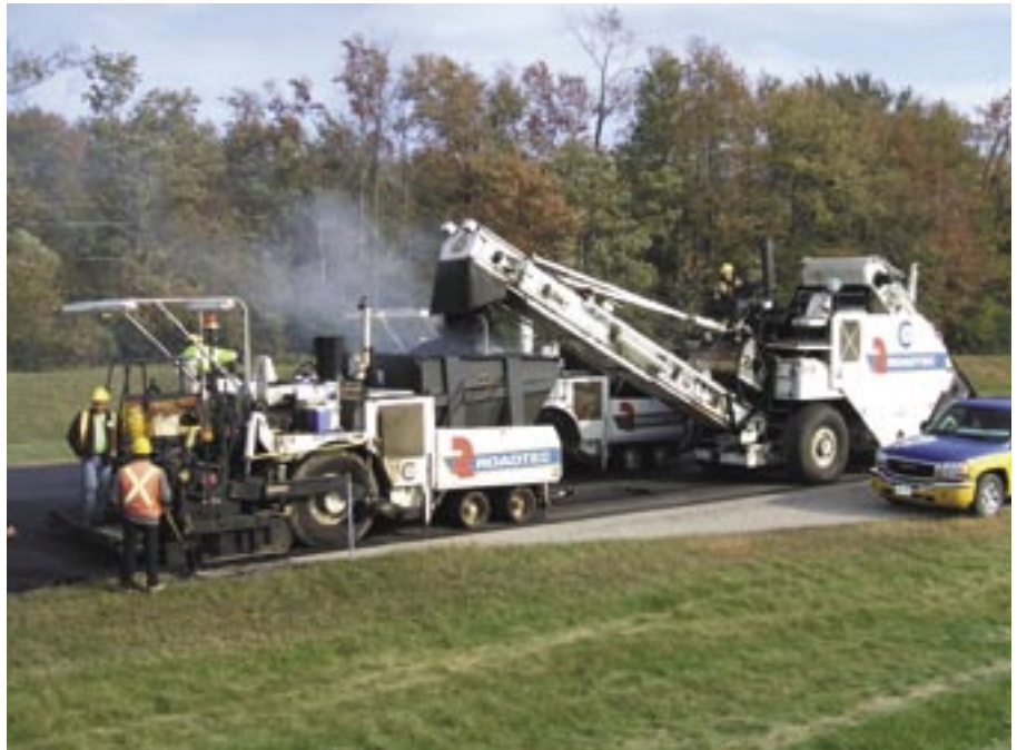
Capital's paving train included a Roadtec SB-2500C Shuttle Buggy feeding a Roadtec RP190 paver. The paver was equipped with a 10-20 Hydraulic Screed, MOBA electronic grade package, non-contacting ski, fully automated feed package, electric screed heater and custom/in-house lighting package.
